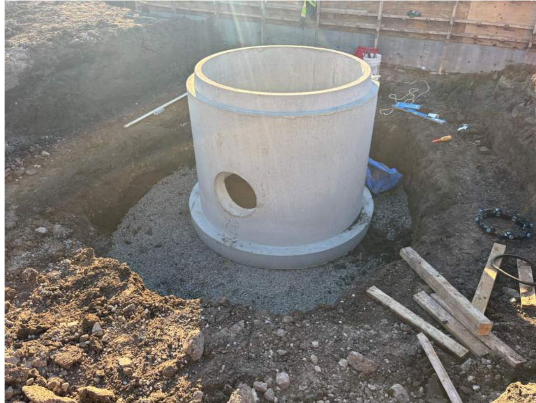
Site Valve Vault
