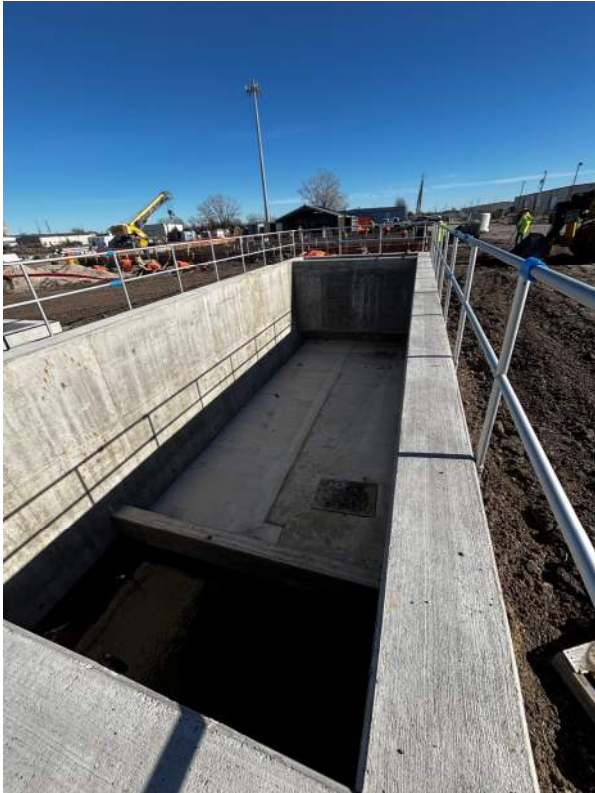
Backwash Settling Tank
